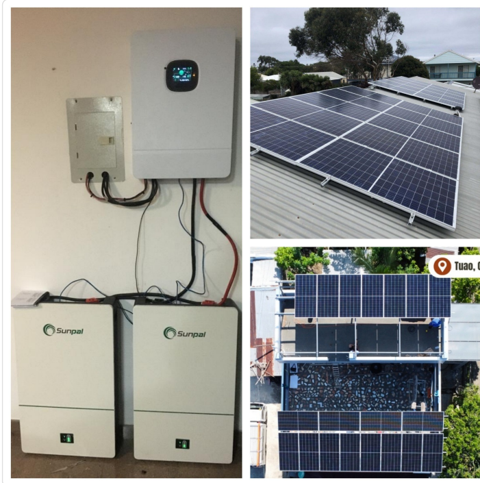
Wall-mounted hybrid inverter with battery storage, and rooftop-mounted solar panels — installed and commissioned as part of a completed system deployment
