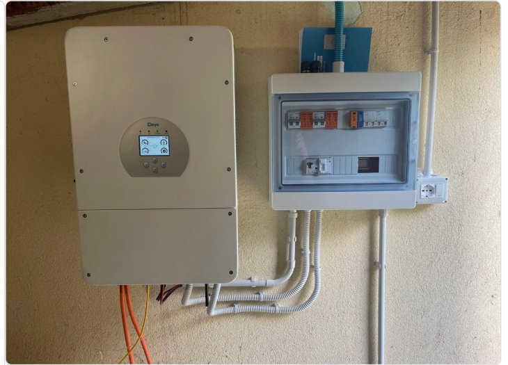
Wall-mounted hybrid inverter and protection/distribution panel, wired and commissioned on site
